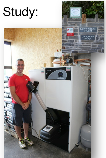
Hywel Davies next to the newly installed Varmebaronen 20kw pellet boiler.
